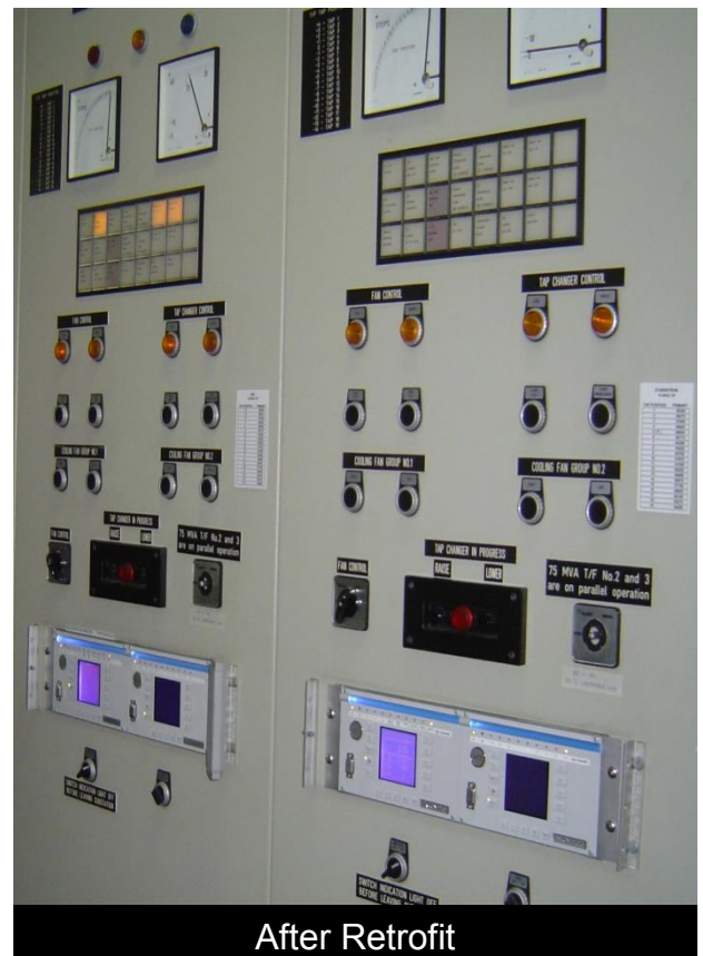
66/22kV 75MVA Transformer
