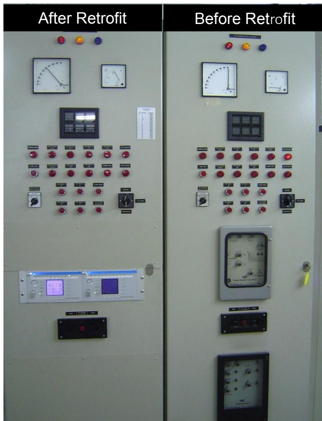
66/22kV 31.25MVA Transformer
